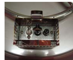
Top View- note next to burner
